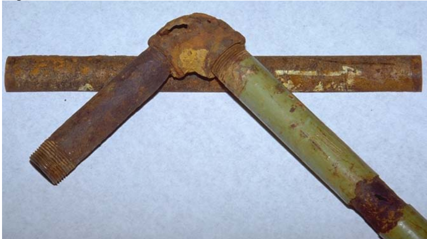
Figure III-23 Poor Construction Practice
